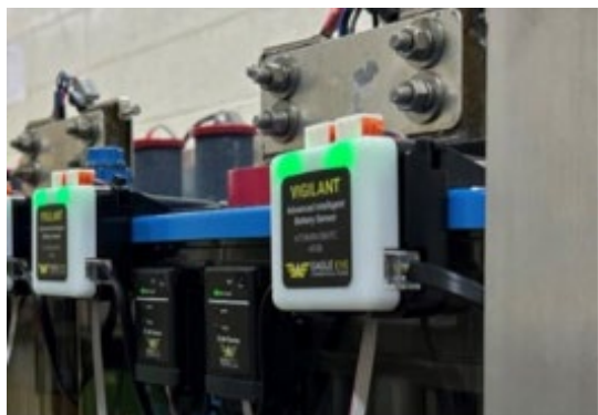
An automated battery backup system installed on the station service battery at Glen Canyon Powerplant, Arizona.
