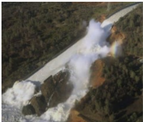
Hydraulic jacking failure at Oroville Dam, California, in 2017.
