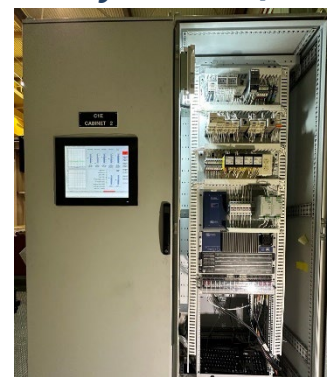
New voltage regulator control system at Fontenelle Powerplant, Wyoming.
